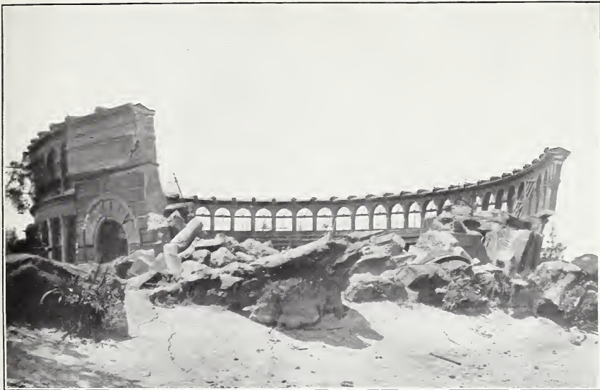
A. EARTHQUAKE EFFECT ON STRUCTURE OF REINFORCED CONCRETE OF POOR QUALITY. Cyclorama, Strawberry Hill, Golden Gate Park, San Francisco. Photograph by Richard L. Humphrey.
